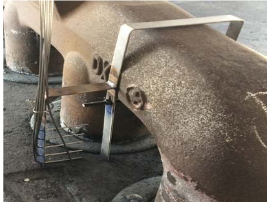
Figure 3. Thermocouples above the anode, fixed to the yoke.
